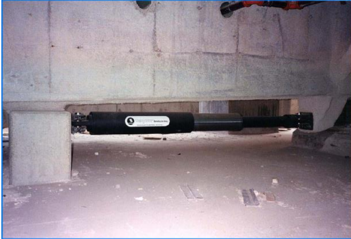
Viscous damper in a building
