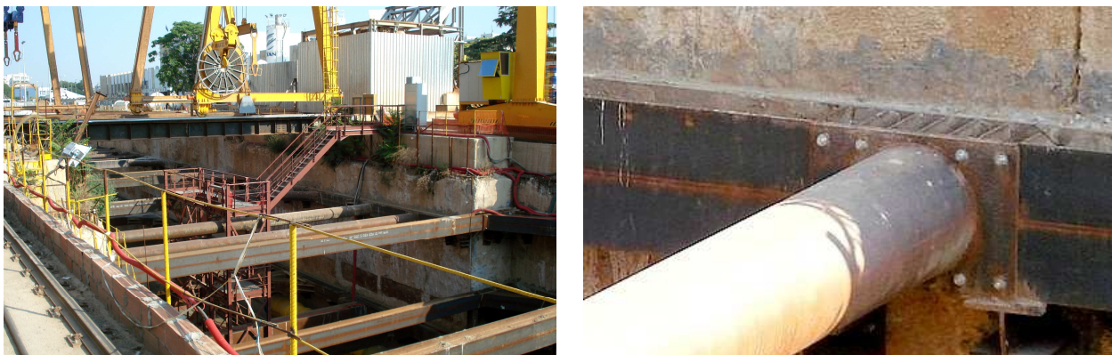
Figure 30-7 Cofferdam for the construction of the metro line in Thessaloniki, with bolt connections struts-wales (August 2009)
