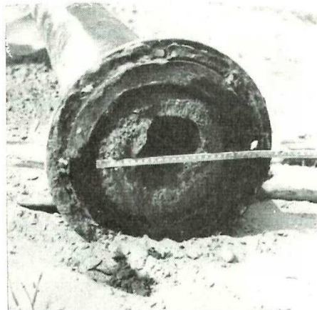
Figure 41-3 Blocked pipe used during construction of the Haringvliet discharge sluice in the building pit
