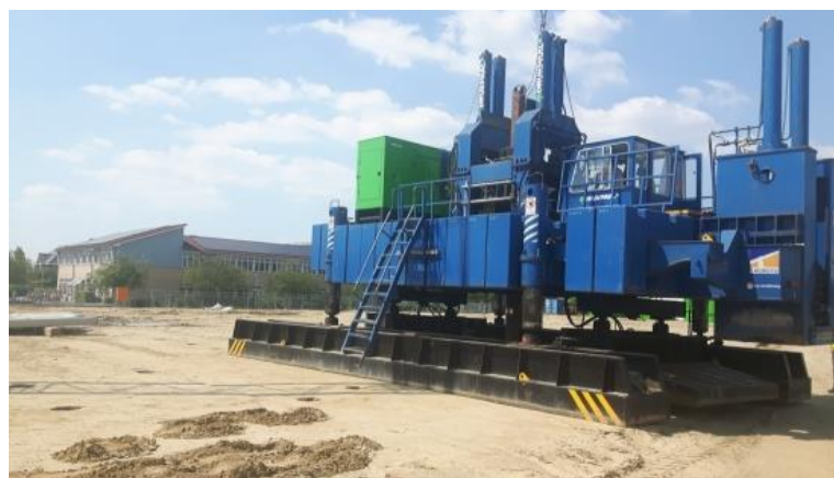
Figure 2.3b Press-in piling for precast concrete piles (used for example in project Sebastiaansbrug Delft, 2019, drukpaal.nl)
