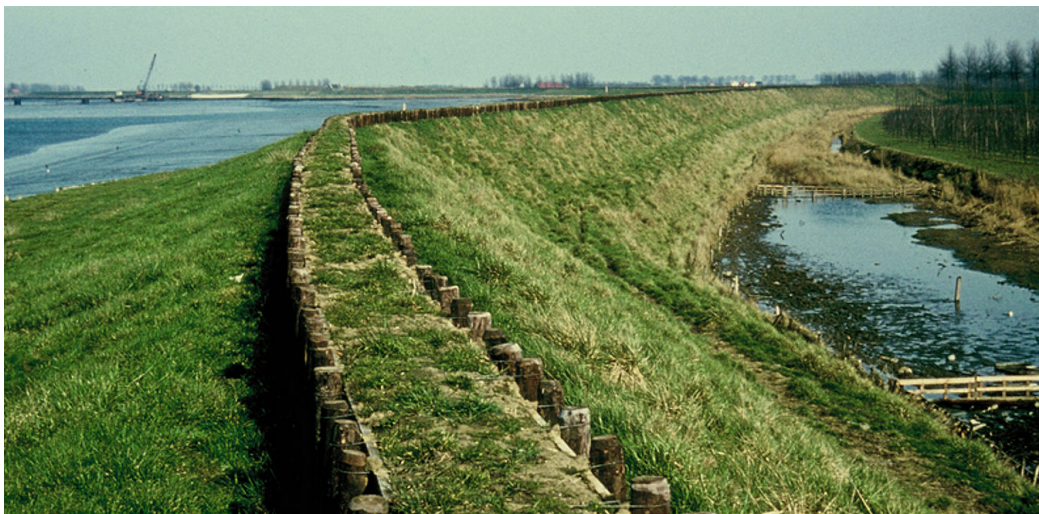
Figure 1.71: Cofferdam wall in a dike in Zeeland to increase the flood retaining height (RWS, 1968)
