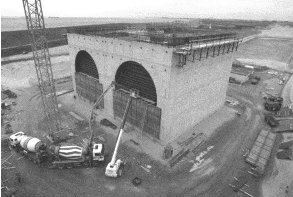
Figure 4.9: Entrance shaft of the Westerschelde tunnel constructed as a caisson at ground level)
