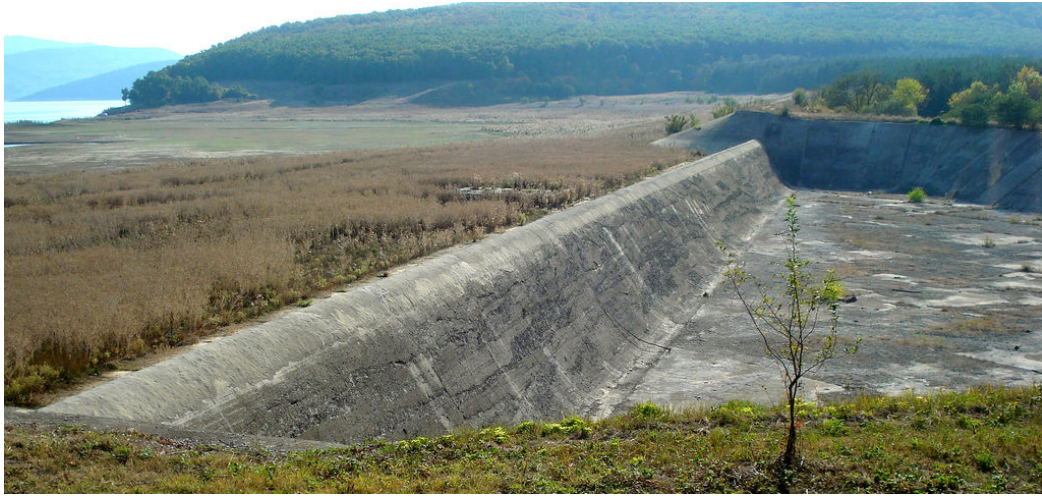
Figure 1.40: Spillway near the Tsonevo reservoir dam in Bulgaria, during the dry season (TU Delft, 2011)
