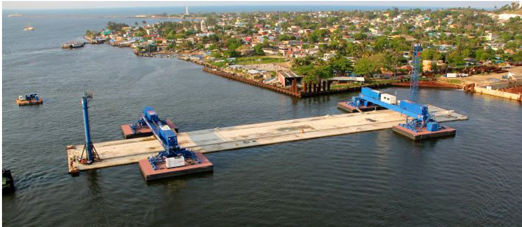
Figure 1.48: Positioning of a tunnel element for the Coatzacoalcos Tunnel Mexico (Volker Wessels, 2013)
