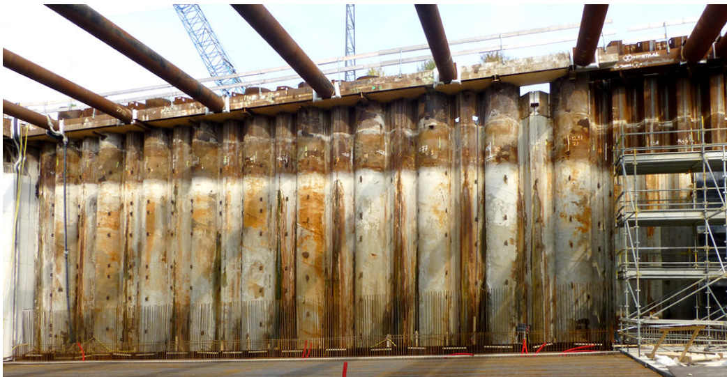
Figure 1.72: Combiwall for the start shaft of the tunnel bore machine for the Rotterdamse Baan, Den Haag (TU Delft, 2018)
