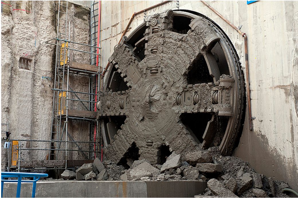
Figure 1.50: Break-through of a TBM in a head wall for a train tunnel, East London ( www.ianvisits.co.uk )
