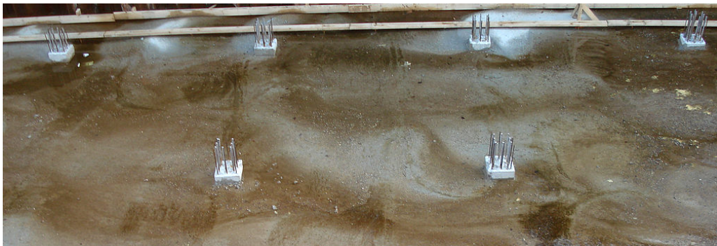
Figure 1.64: Underwater concrete and tension piles in the approach to the railroad tunnel near Kampen (Hanzelijn) (TU Delft, 2007)
