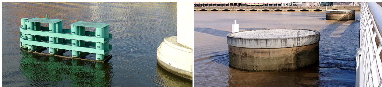
(a) Steel collision structure in front of a bridge pier in the Oder near Szczecin, Poland (TU Delft, 2017) (b) Concrete collision structure in front of the lift-bridge over the Garonne near Bordeaux, France (TU Delft, 2019)
