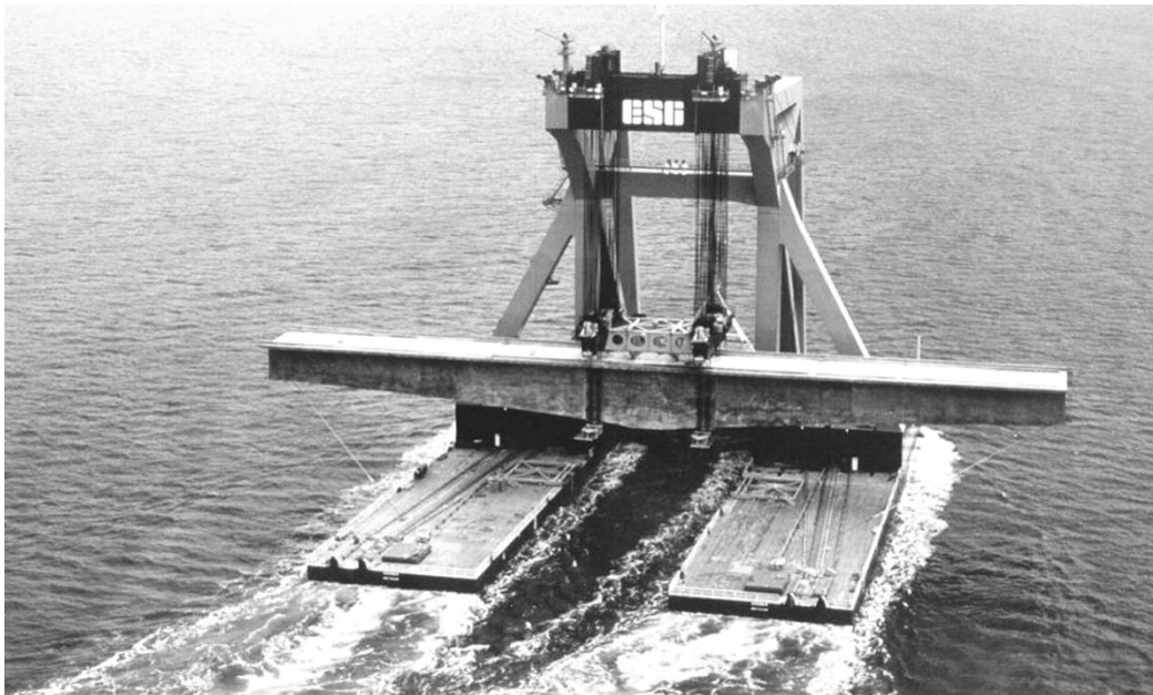
Figure 5.4: Floating crane Svanen (Ballast Nedam) with bridge girder for the Westbridge over the Great Belt, Denmark
