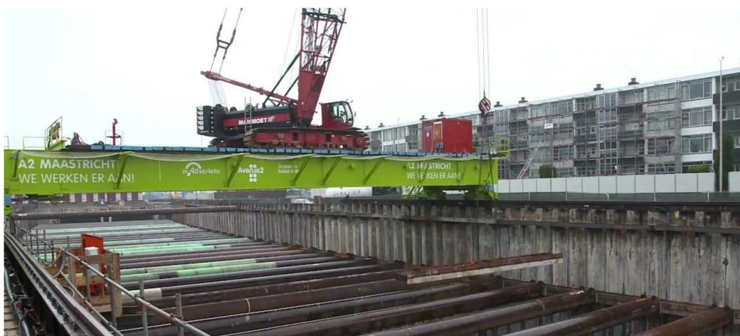
Figure 1.60: Cofferdam with a framework of wales and struts, and a traverse for the road tunnel in Maastricht (Avenue2)
