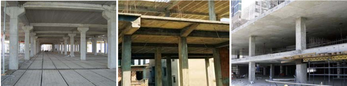
Fig. 14. 3: Structural types of slabs a) one-way slab with line supports, b) two-way slab with line supports and c) flat slab
