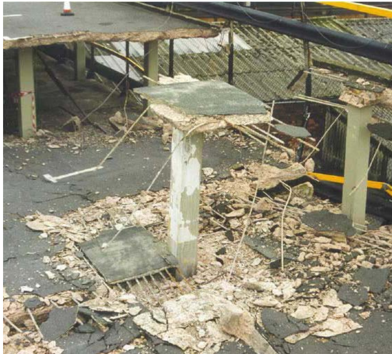
Fig. 14. 76: Punching shear failure mechanism in a flat slab and the functioning of shear reinforcement (if required) (top) and an example of the actual failure of a flat slab
