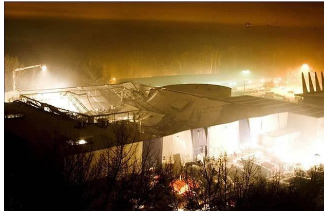
Figure 10.12 Collapse of the roof of the Katowice International Fair due to snow load (Wikipedia)
