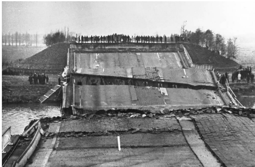
Figure 10.6 This bridge over the highway 'Boudewijn' in Pulle collapsed (1966) due to erosion of the east bank in the vicinity of the pile foundation at the side of the canal Nete
