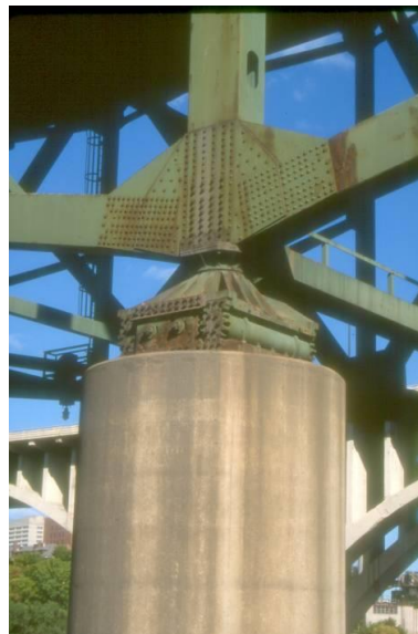
Figure 10.14 Under-sized gusset plate of I-35W over the Mississippi (Wikipedia)
