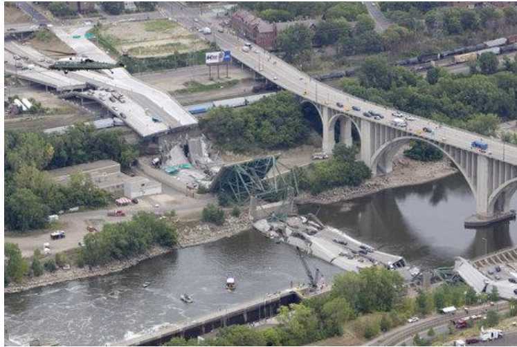
Figure 10.13 Collapse of the steel truss arch bridge I-35W over the Mississippi (Wikipedia)
